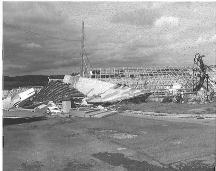
A construction trailer was demolished when it slammed into nearby greenhouses.
